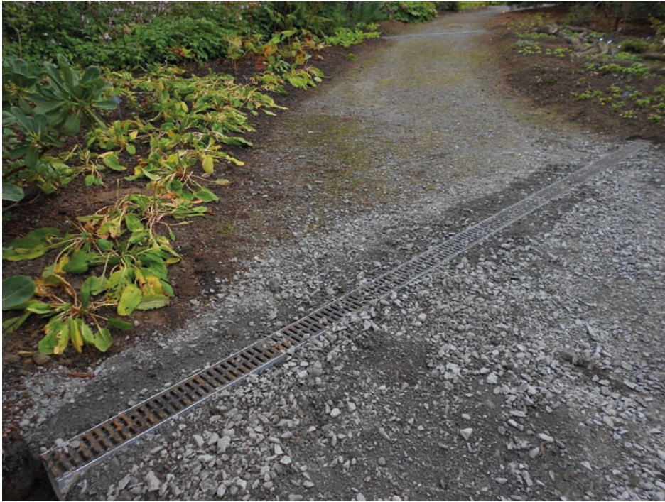
Fig. 2 Resurfaced path and new drainage at RBGE following erosion caused by flooding in July 2012. Photo: David Knott.
