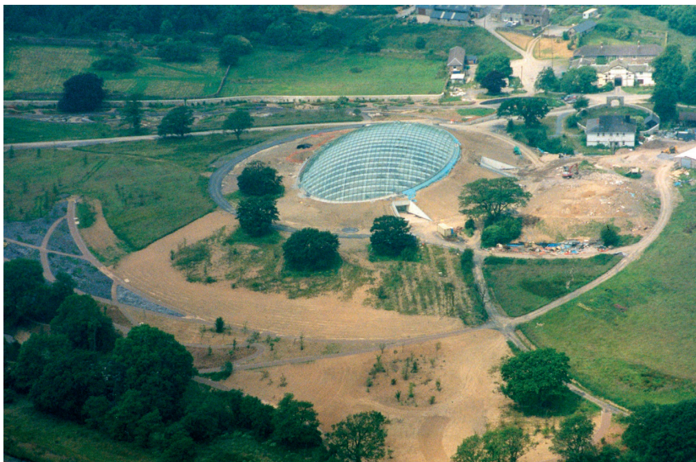
Fig. 3 The Great Glasshouse during the latter stages of construction in 1999 (Photo: National Botanic Garden of Wales).
