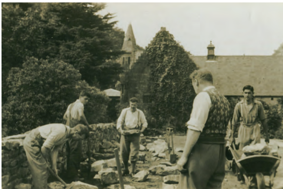
Fig. 19 Black-and-white photo. Construction work supervised by Dr J.M. Cowan, c. 1934. Miscellaneous photograph in Benmore Curator's office, kindly made available by Peter Baxter.
