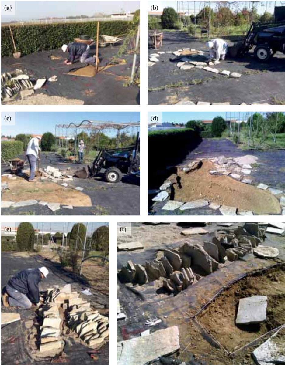
Fig. 4 Basic construction steps followed for the creation of the Ionian Islands Unique Rock Garden: (a): Cutting off the permeable landscape fabric. (b): Setting slate stones of different sizes according to the actual geographical terrain of the Ionian Islands (here Cephalonia). (c): Digging the base for slate. (d): Creation of a base for slate (c. 30cm deep). (e) and (f): Setting slate vertically to simulate the actual geographical relief of each island i.e. Cephalonia (e) and Ithaca (f) (Photos: Marina Panagiotidou).
