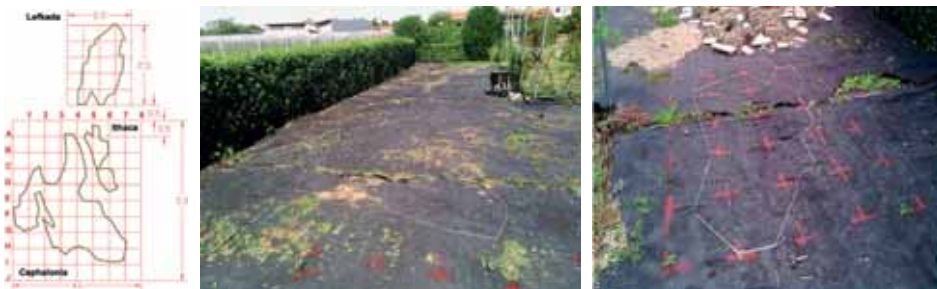
Fig. 3 Transfer of basic design (left) on the site by creating a 50 × 50cm canvas on the ground with red marker in order to imprint and establish the natural shape of Cephalonia (middle) and Lefkada Island (right). Dimensions are shown in metres. Plan and photos: Marina Panagiotidou.
