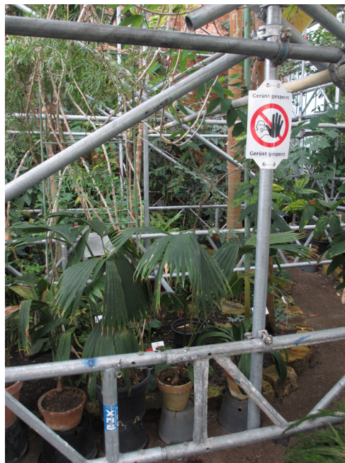
Fig. 9 The advanced corrosion of the footings in the palm house made bracing with scaffolding elements necessary. Fortunately, garden staff could continue to look after the plants, albeit under difficult conditions and with a few 'gymnastics'. Photo: P. König.
