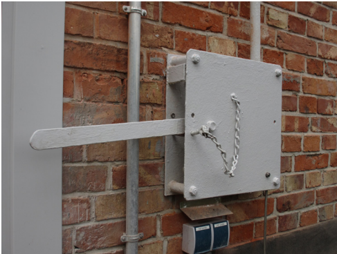
Fig. 12 The existing lever on a ventilation flap was retained and is fully functional. Photo: P. König.
