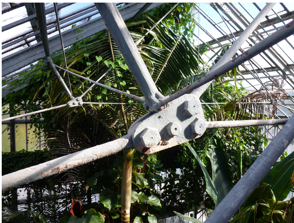
Fig. 3 Reinforcement bracing developed by two engineers, Wiegmann and Polonceau, in the palm house, the largest greenhouse in the complex with a ridge height of 12 m, before restoration. Photo: P. König.
