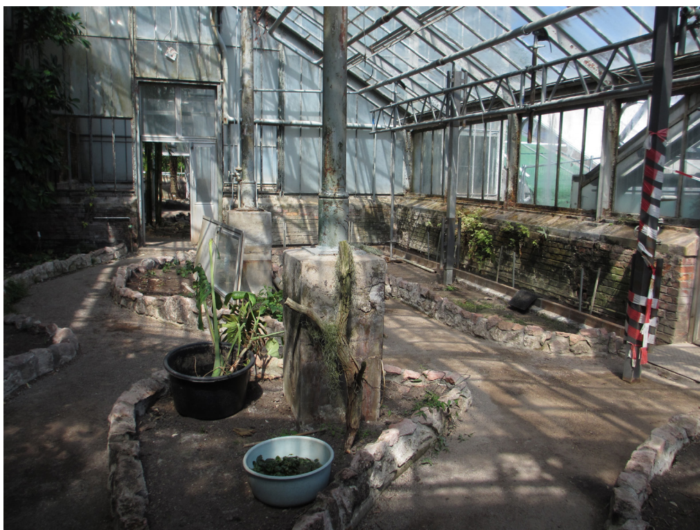
Fig. 14 Almost-empty tropical house: (centre) the two cast-iron supports; (right) the temporary static reinforcement with scaffolding elements. Photo: P. König.
