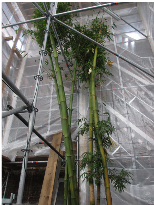
Fig. 15 Bambusa vulgaris , one of seven plants remaining in the greenhouses during the reconstruction work, protected by heated and illuminated polyethylene enclosures. The massive bamboo probably dates back to the early days of the greenhouses. Photo: P. König.
