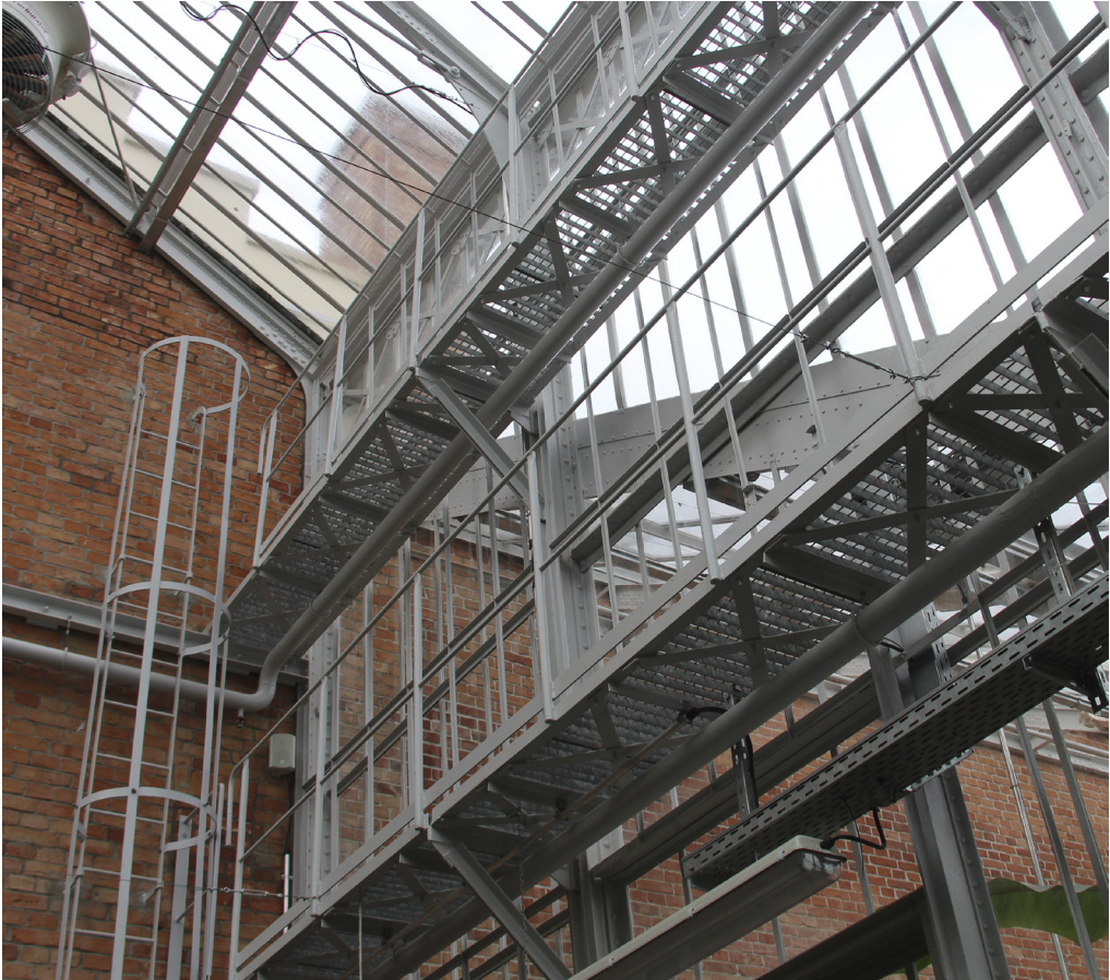
Fig. 4 Palm house, two U-shaped maintenance galleries with access ladder, after restoration and the addition of a safety cage. Photo: P. König.
