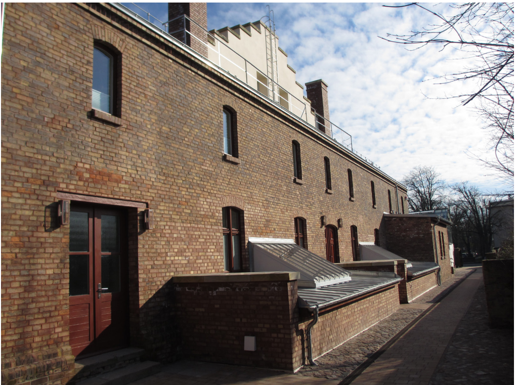
Fig. 17 West view of the service building after the reconstruction. The hatches, which are now glazed, were formerly used as coal chutes. The gable of the palm house can be seen in the upper part of the photo. Photo: P. König.
