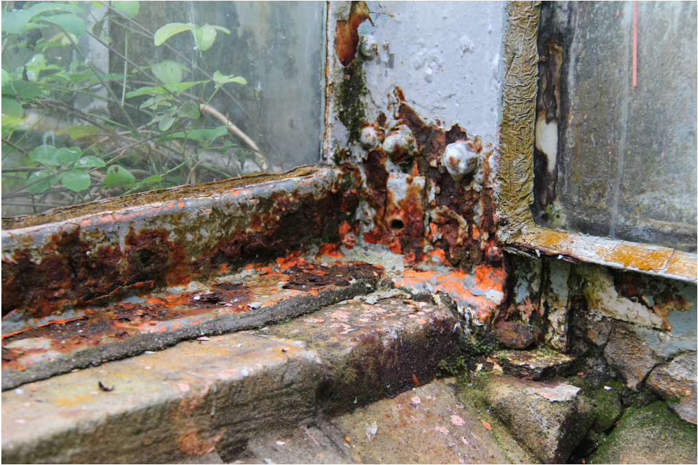
Fig. 7 Corrosion and rust damage at the base of the frame construction. Photo: P. König.
