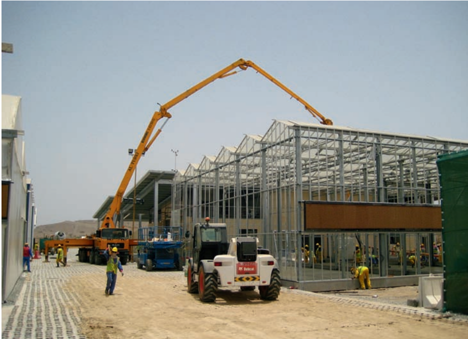
Fig. 3 Towards the final stages of Oman Botanic Garden nursery construction. Concrete is being pumped in to form the floor of the Propagation Glasshouse in July 2008. Photo: Leigh Morris.
