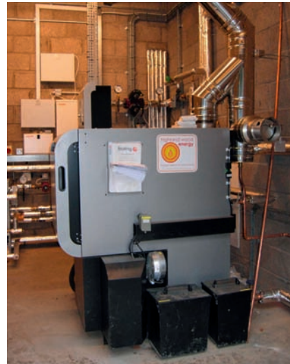
Fig. 5 The biomass boiler provides heat by burning woodchips sourced from locally grown trees. Photo: David Knott.
